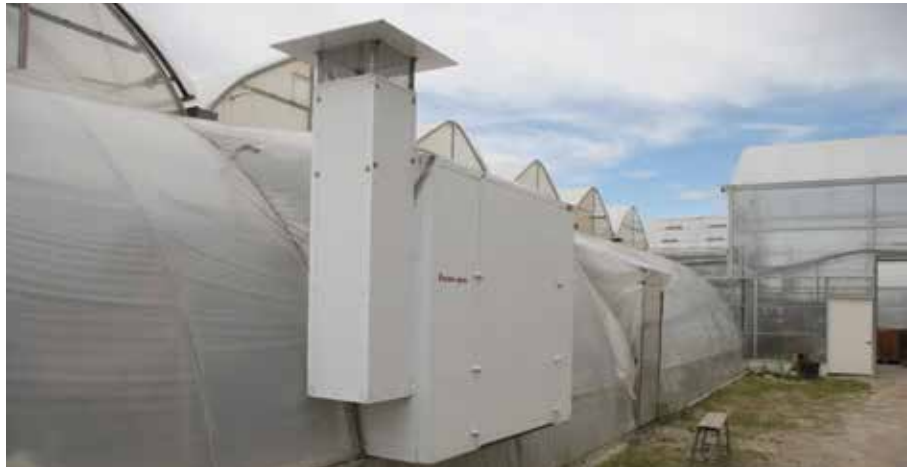
The Heemans recently installed a heat exchanger on their main retail greenhouse.
