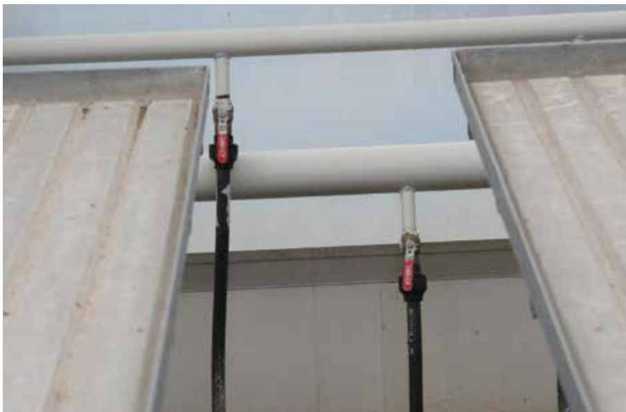
An example of the water lines for the in-floor heating system at the Heeman greenhouse operation.
