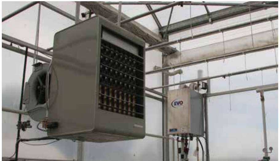
The forced air furnace to the left is 250,000 BTU. To its right is the gas-powered water heater. That little box is 600,000 BTU. “That’s heating the water (for the Heeman greenhouse’s in-floor heat) and that’s 99 per cent efficient,” says Rudy Heeman.
