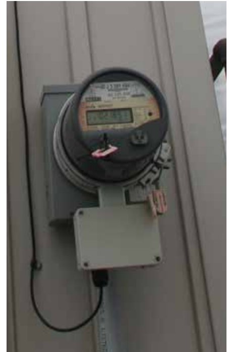
The digital hydro meter at the Heeman farm is unable to transmit readings to the utility.
